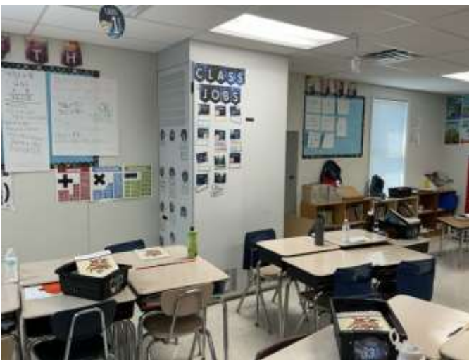
33 - TYPICAL MODULAR CLASSROOM / HEAT PUMP
