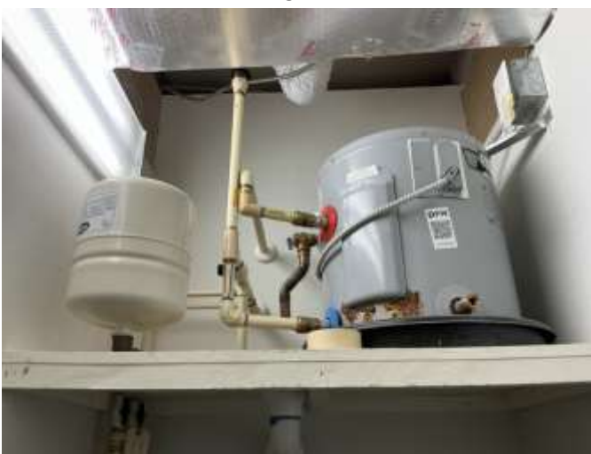
35 - MODULAR BUILDING WATER HEATER
