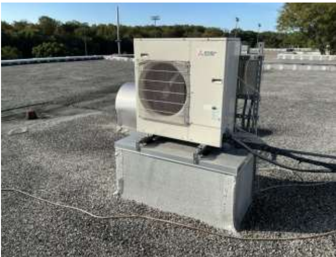
27 - SUPPLEMENTAL HVAC EQUIPMENT
