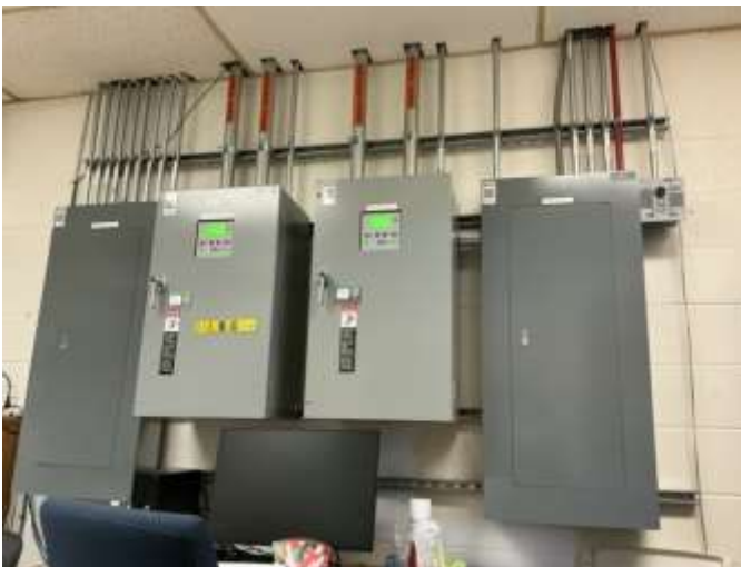
21 - ATS / DISTRIBUTION PANELS
