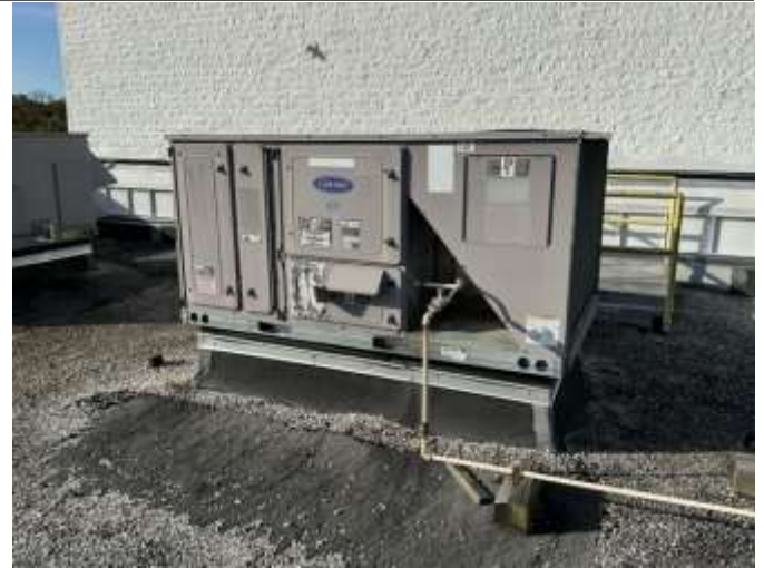
26 - PACKAGED ROOFTOP UNIT
