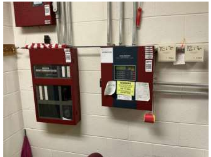
28 - FIRE ALARM PANEL
