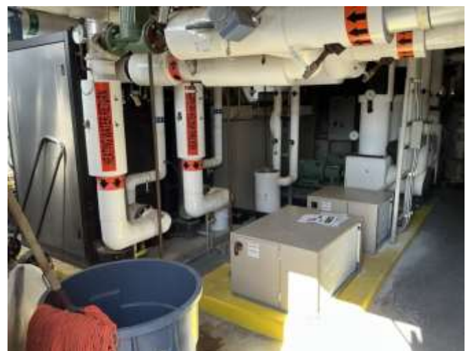
24 - MAIN MECHANICAL ROOM
